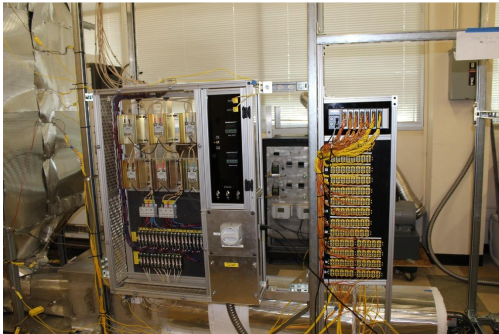
Figure B.7. Heater control system (left) and thermocouple board (right).
